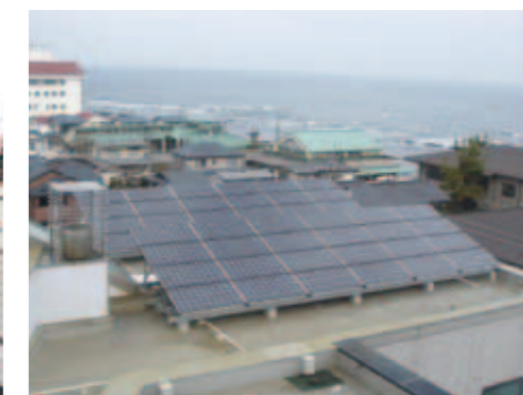
Solar power generator installed on the roof of a government building (Hirono Town)
