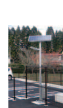
Solar power generator at a daycare center (Noda Village)
