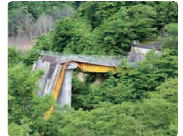
The bridge collapsed at nearly a right angle because of the pressure from the shifting ground
