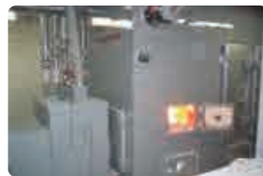
A pellet boiler
