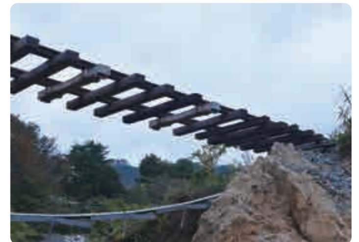
The railway tracks left hanging in the air after the typhoon in the Funakoshi area of Yamada Town
