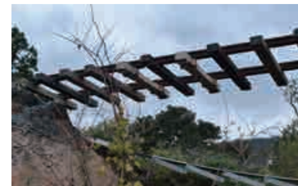
Roads were severely damaged by the East Japan Typhoon. Photo of the Sanriku Railway tracks, after the roadbed was washed away.
