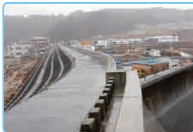
Earthquake Disaster Remains: The Taro Seawall. The first seawall extending to the back and the damaged second seawall continuing to the right
